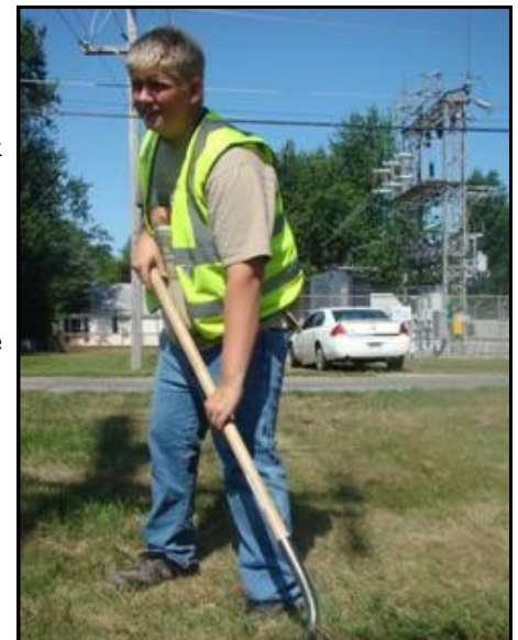
Logan Sherman, digging grass away from a drain pipe in the Village of Breckenridge.
